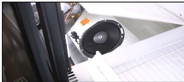
Fig. 96 Running evaporator fans
