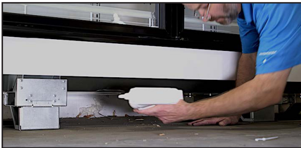
Fig. 49 PVC drain oriented left toward grease trap.
