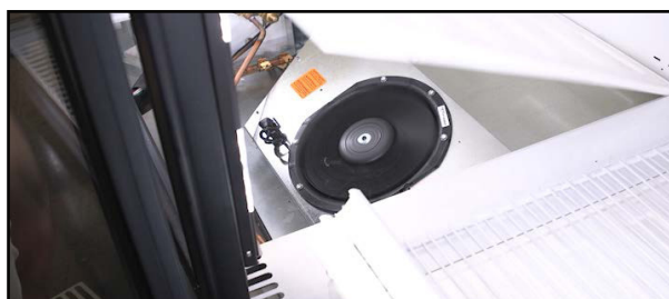
Fig. 94 Running evaporator fans
