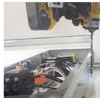
Fig. 82 Secure electrical junction box
