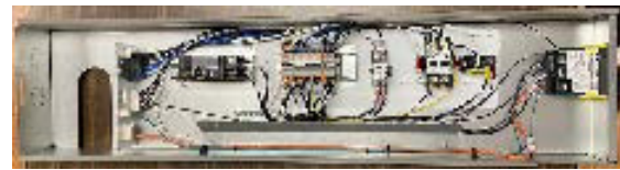
Fig. 98 Electrical Junction Box
