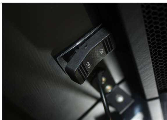
Fig. 10 Upper cornice light switch
