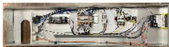
Fig. 98 Electrical Junction Box
