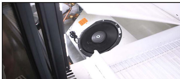
Fig. 94 Running evaporator fans
