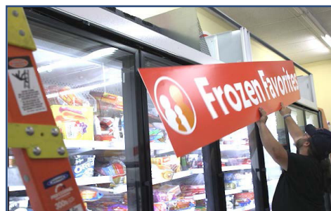
Fig. 88 Mount store signage to fascia
