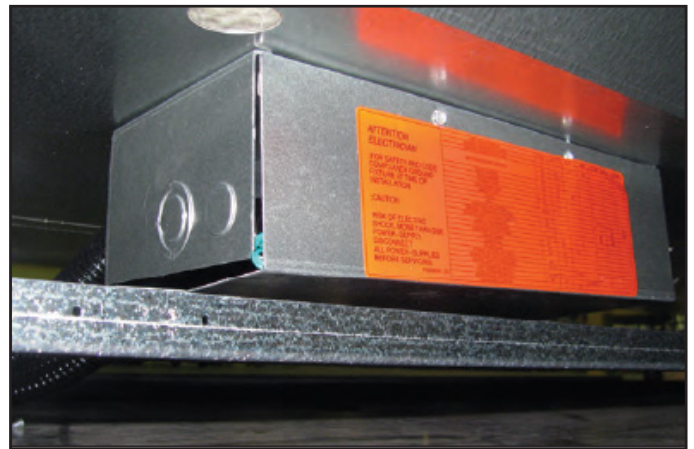
Fig. 10: Junction box beneath case
