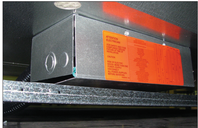
Fig. 14 Junction box beneath case
