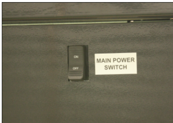
Fig. 10 Lower panel power switch
