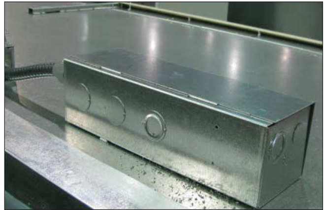
Fig. 12 Junction box on top of case
