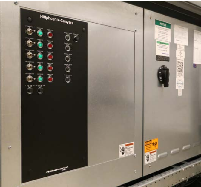
Main control panel
