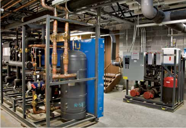
Second Nature® system and pump station
