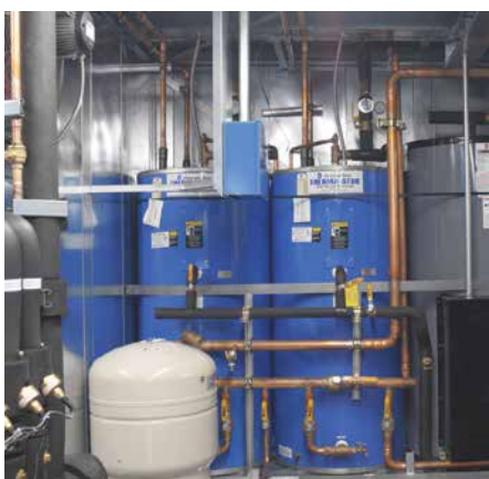
You can use up to 100% of the available waste heat from your system.
