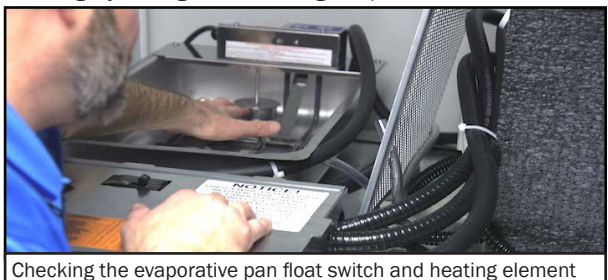
Checking the evaporative pan float switch and heating element
