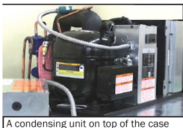
A condensing unit on top of the case
