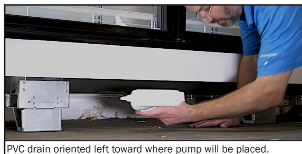
PVC drain oriented left toward where pump will be placed.
