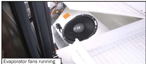
Evaporator fans running
