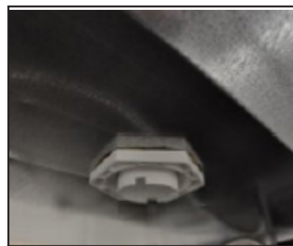
Avoid the drain hub when using a pallet jack
